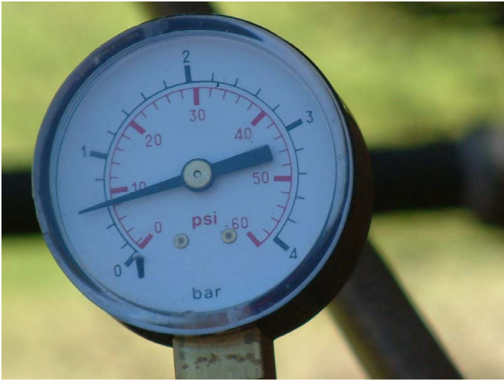
PRESSURE METER DISPLAYING THE READING OF 0.5 BAR
